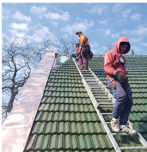
At left: 100-year old clay roofing tiles that were cracked and failing were replaced in 2023-24 as part of the church's 2014 Reserve Plan and 2018 Capital Fund.
